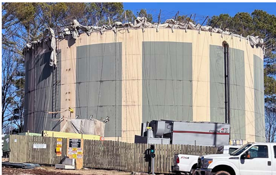
TANK'S FUTURE HALF FULL? The massive water tank that has loomed with omnipresence for decades at the corner of Sparkman Drive and Pulaski Pike is finally getting some tender loving care, according to Huntsville Utilities Gary T. Whitley, Jr., who sees a bright mural in its future. [Photo: Saintjones]
